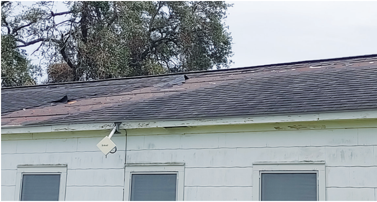
Danevang Lutheran Church, Danevang, TX: roofs of three church buildings were damaged by Hurricane Beryl.
